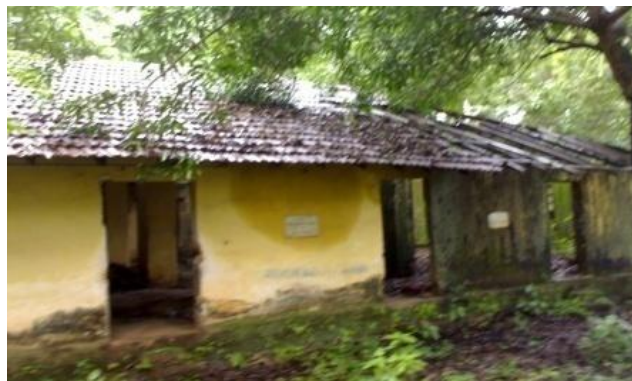
Dilapidated condition of leprosy hospital
